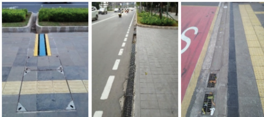
Figure 3. Holes from Roads and Pedestrians' Paths are Too Small
