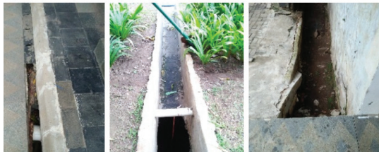
Figure 4. The Small Trench Cover is also Blocked by Litter
