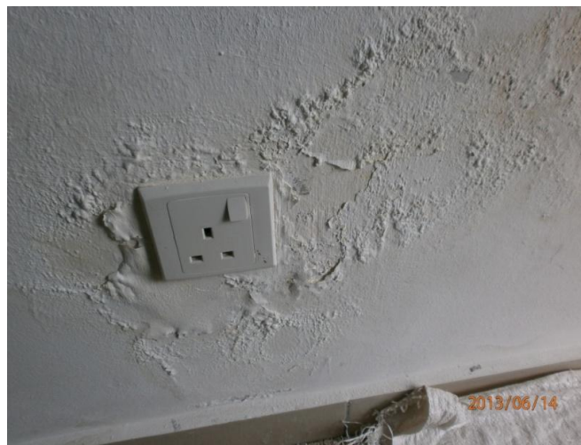
Figure 3.7 Peel of paint (dampness)
