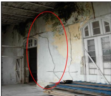
Grid: B/7-8 (Y3), Checklist 37 Photo: Minor Cracks Along Wall Plaster
