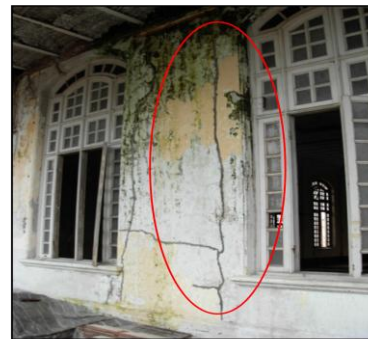
Grid: B/9-10 (Y4), Checklist 38 Photo: Vertical Cracks
