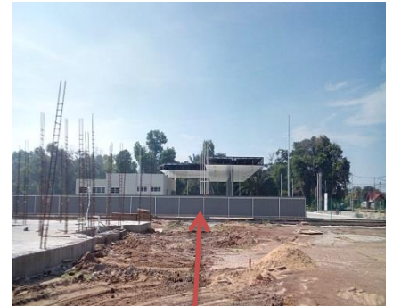
Photo 3.4.3.3: pump station (CALTEX)
