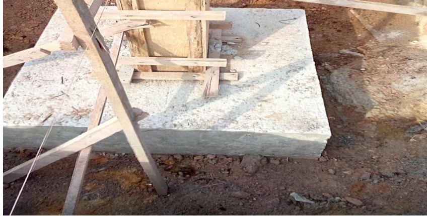
Photo 3.7.9: Hardens Pad Footing
