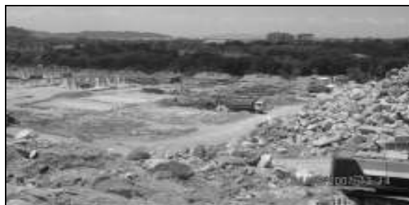
Fig. 1 Soil erosion on a construction sites
