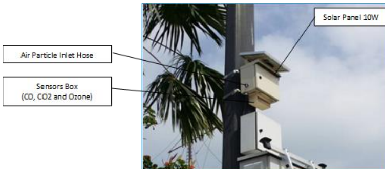
Figure 6: Set of RTU with gas sensors set up on a pole
