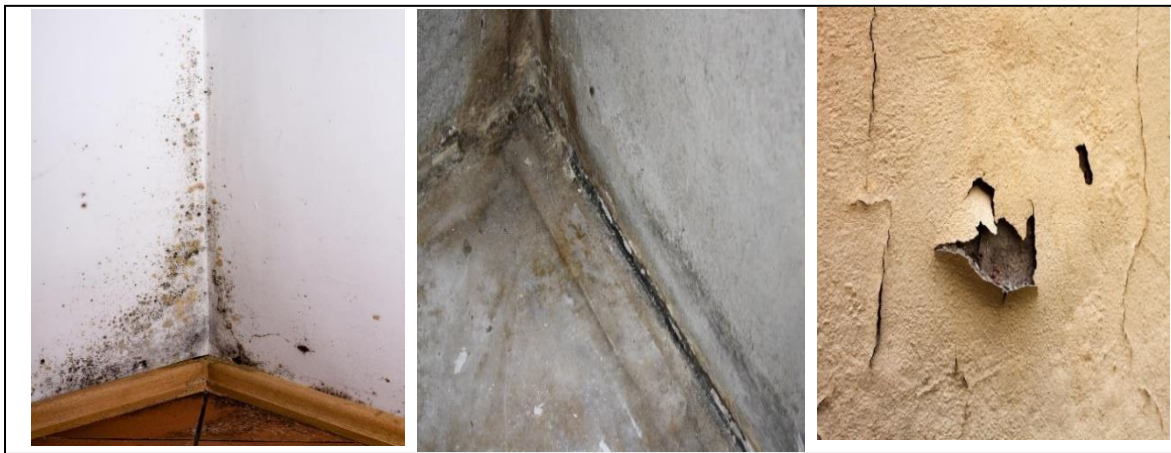
Figure 1: The example of building defects occurs at building due to high humidity (Source: Halim et al., 2012)
