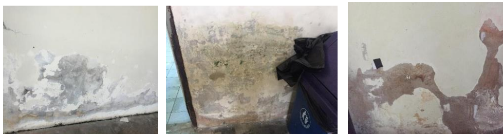
Figure 6: Example taken from a pilot study of this study: Rising damp at Student's accommodation, UiTM Perak.
