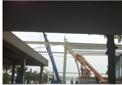
(b) Crane works without proper safety equipment
