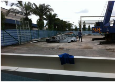
(c) Working without safety equipment
