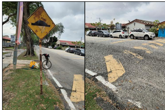
Plate 5.50 Speed Hump for Traffic Calming at SK Seksyen 24
