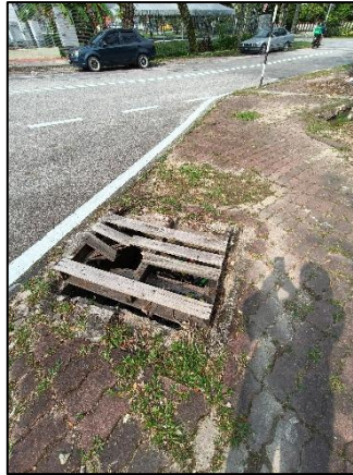
Plate 5.73 Hazardous Obstruction at SK Jalan U3
