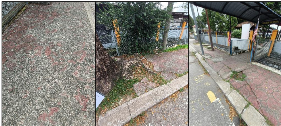
Plate 5.21 Poor Surface Condition of School Walkway at SK Seksyen 17
