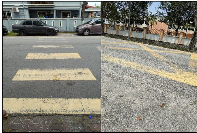
Plate 5.37 Faded Crosswalk Markings at SK Seksyen 19
