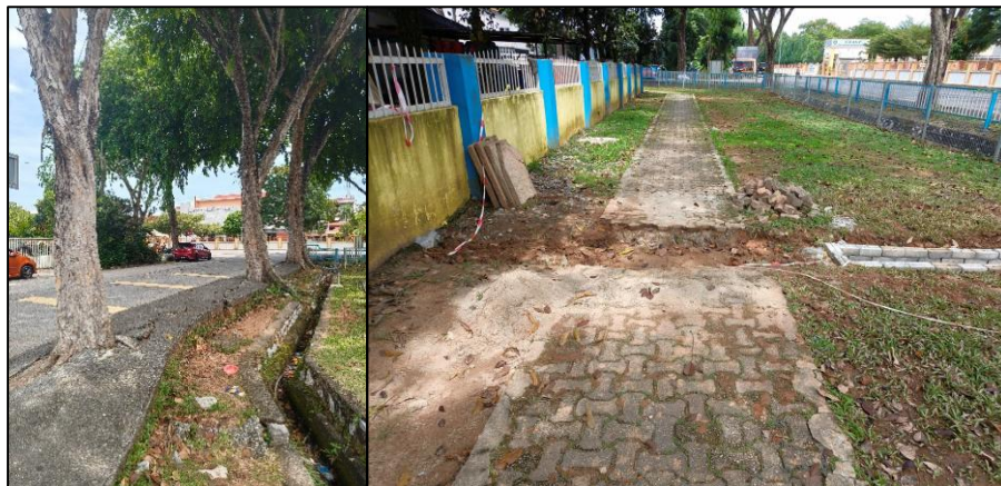
Plate 5.36 Obstructions at SK Seksyen 19
