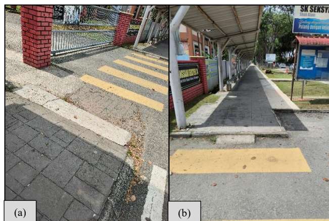
Plate 5.47 Non-Compliant Curb Ramp at SK Seksyen 24
