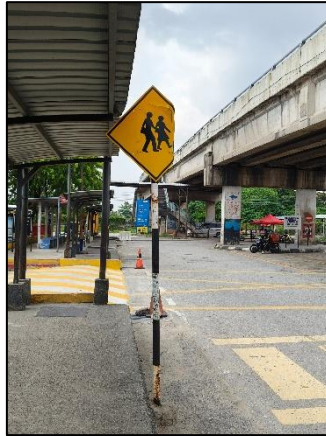
Plate 5.64 Damaged Signage at SK Padang Jawa
