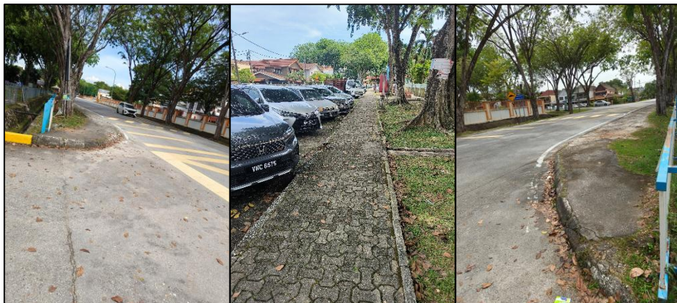
Plate 5.34 Damaged and Poorly Maintained Pedestrian Surface at SK Seksyen 19
