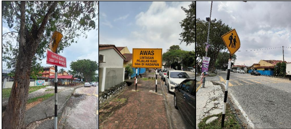
Plate 5.51 Damaged and Inadequate School Signage at SK Seksyen 24
