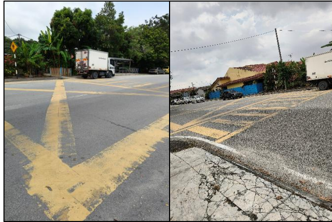
Plate 5.49 Faded Crosswalk Markings at SK Seksyen 24
