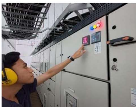
Figure 1: Taking Electrical Supply Readings on the MSB
