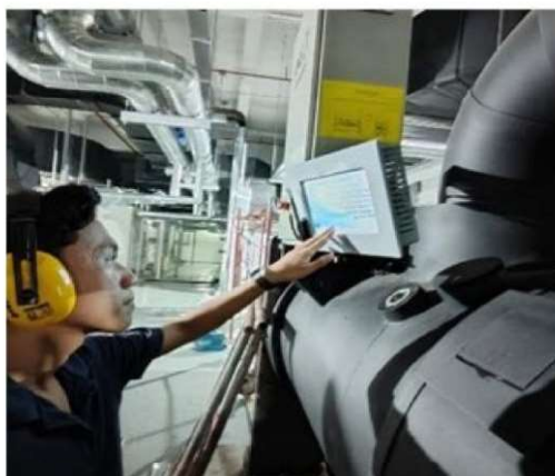
Figure 2: Taking the Chiller Reading
