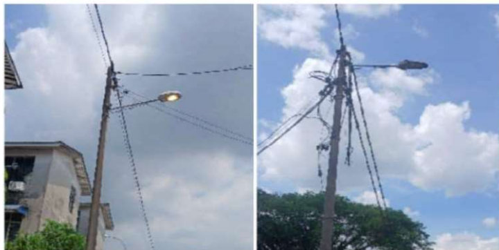
Figure 3: Cable Sagging During Installation
