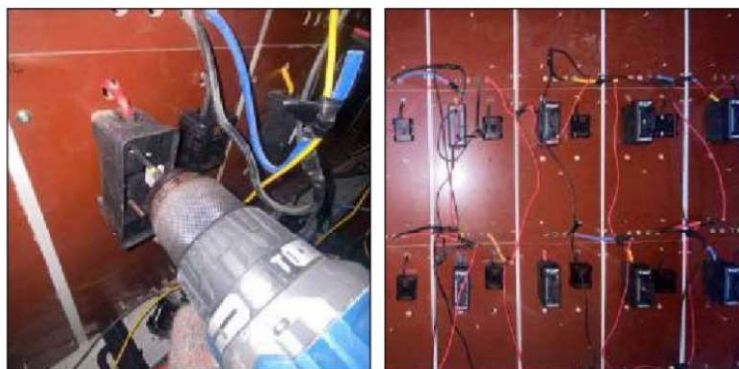
Figure 1: Distribution Meter Board Installation
