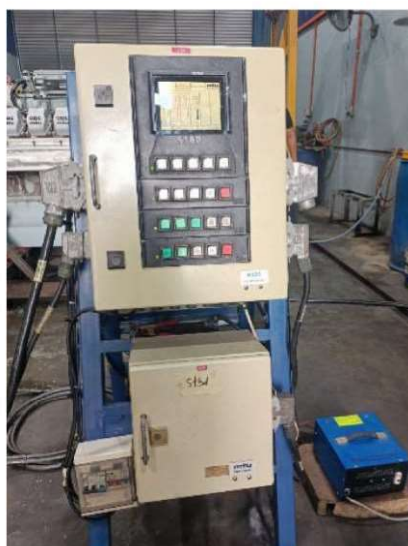
Figure 1: Local Operating Panel (LOP) Used for Engine Control and Monitoring
