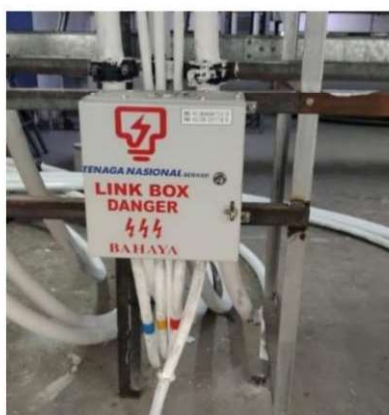
Figure 4: TNB Link Box
