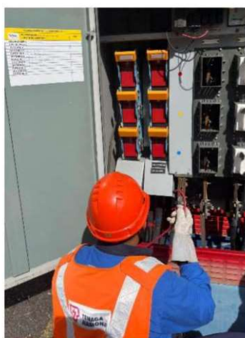
Figure 1: Voltage And Current Measurement at Feeder Pillar During Site Inspection
