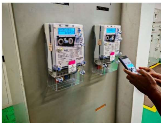
Figure 1: Getting a Close Up Look at Smart Metering Technology (Itron SL7000 Smart Meter) and Learning How to Use Mobile Integration to Verify System Performance
