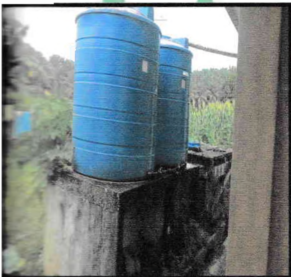
water tank that provide to store a water
