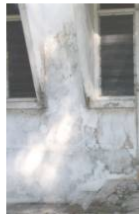
Figure 4d. Stain and crack peeling of paint
