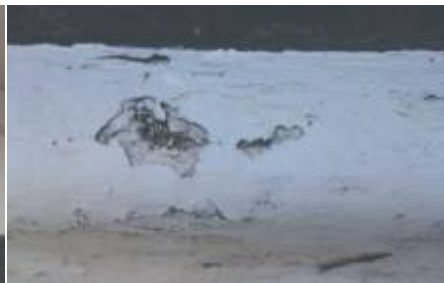
Figure 4f. Blistering of paint and holes
