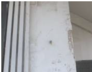
Figure 4e. Cracks in column
