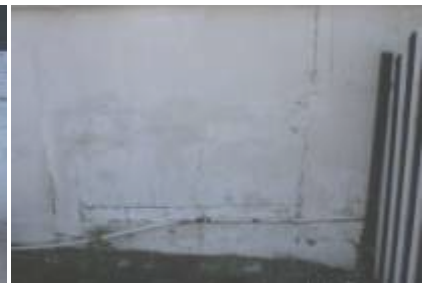
Figure 4g. Crack and stain
