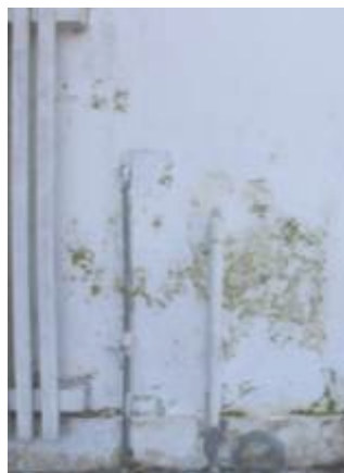
Figure 4c. Greenish stain and peeling of paint
