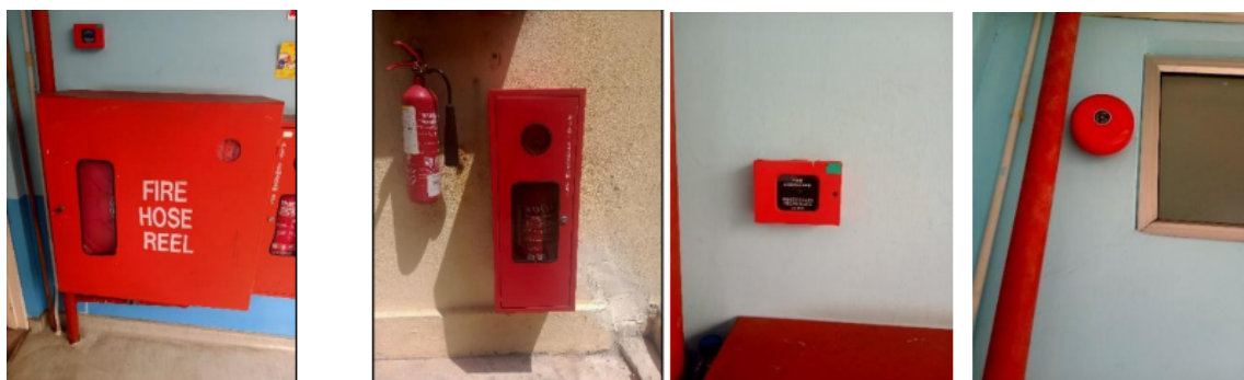
Figure 0-13: Fire hose reel, fire extinguisher and Emergency break glass panel
