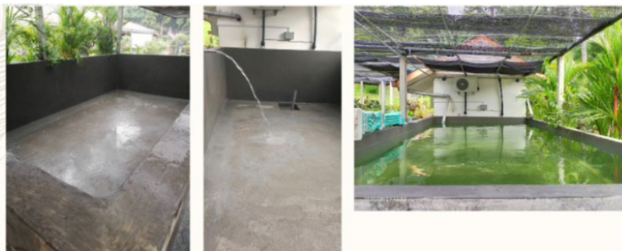
Rainwater being collected in the detention pond before being used for irrigation purposes
