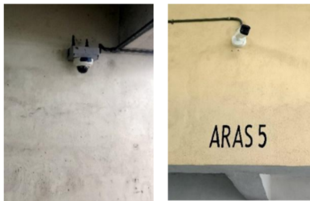
Figure 1.17: Closed circuit television (CCTV)
