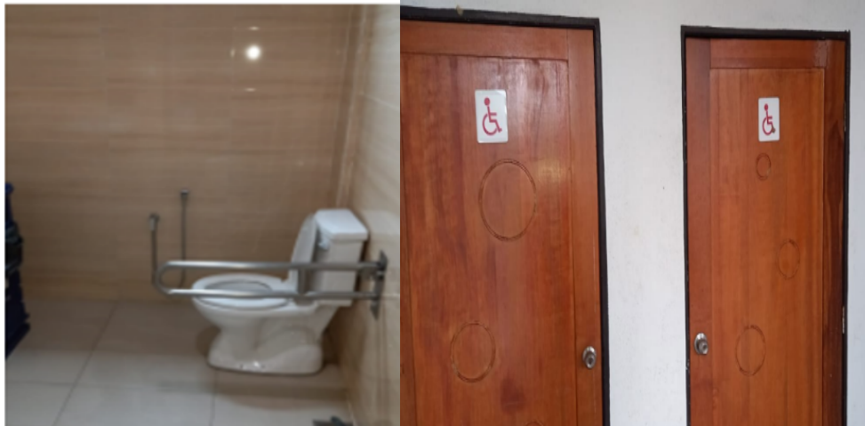
Figure 0-12: Designated toilet for disabled and special needs at Dewan Agong Tuanku Canselor, UiTM Shah Alam
