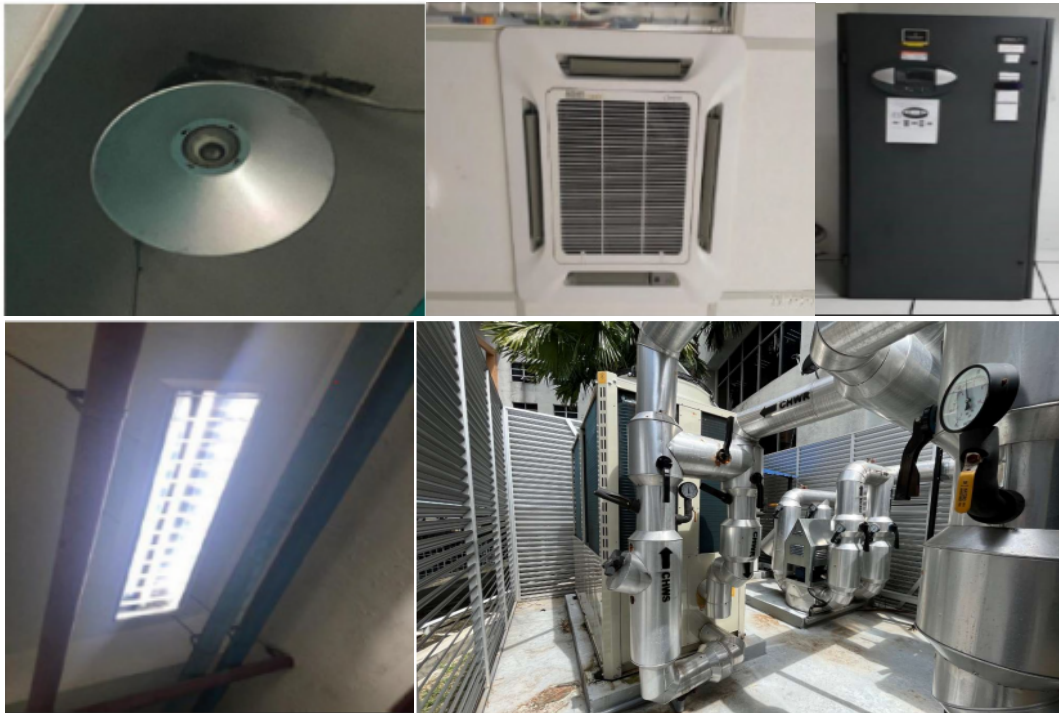
Figure 0-3: Highly Efficient Hybrid Modular Chillers were installed for independent operation time of the cooling system in two Libraries: PTAR 3(80 RT) and PTAR 4 (120RT).
