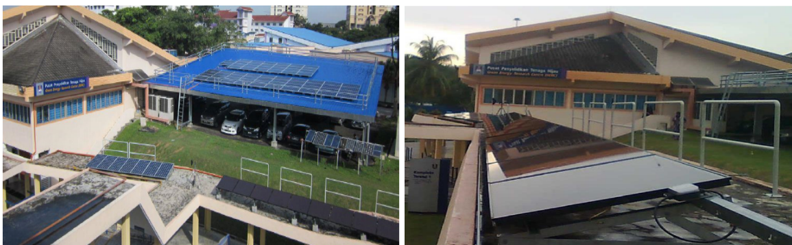
Figure 0-8: 19 kWp Solar PV System (GERC) – Kolej Teratai
