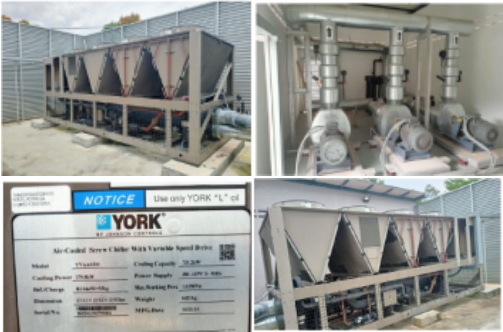
Figure 0-4: Two (2) new chillers were installed with the same capacity. Only one operating at a time, another on standby mode
