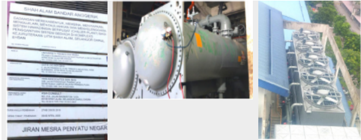
Figure 0-5: Replacement of four (4) RT water-cooled chillers is the major project for energy saving at the Engineering Complex
