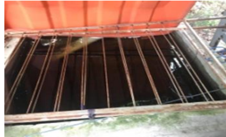
Figure 23 Rainwater harvesting system in UiTM Shah Alam
