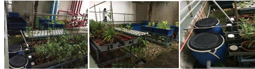
Figure 24 Water recycling system for hydroponic plants at Engineering Complex
