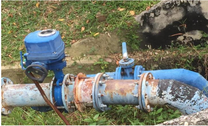
Figure 26 Manual-sensor to control volume of water from SYABAS to pump house UiTM
