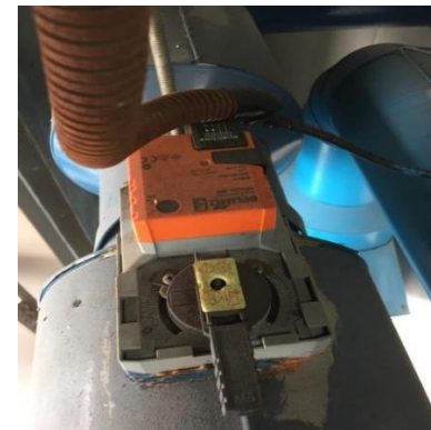
Figure 25 Auto-sensor to control volume and flow of water in the chiller and air-conditioning systems
