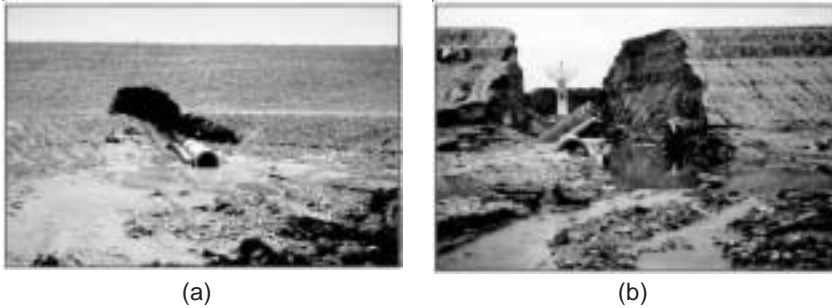
Figure 1: A failure due to internal erosion which leaves a huge void space along the conduit and embankment failure due to discontinuity represented by the conduit. [Photo extracted from Federal Emergency Management Agency (FEMA), National Dam Safety Program, USA – conduit through embankment dam]
