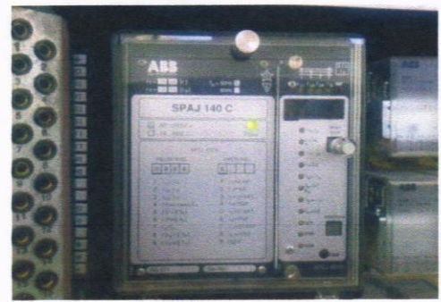
Figure 5: Overcurrent Relay Type SPAJ 140C
