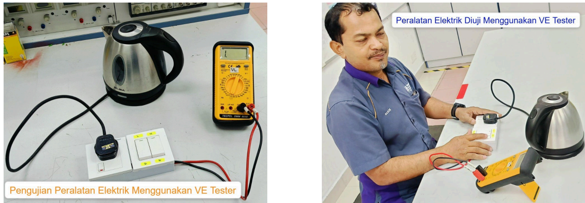
Figure 5. Checking using VE Tester
