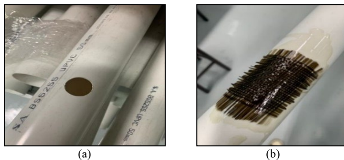
Fig. 3. (a) Defect pipe and (b) PVC pipe patching with woven basalt fiber.
