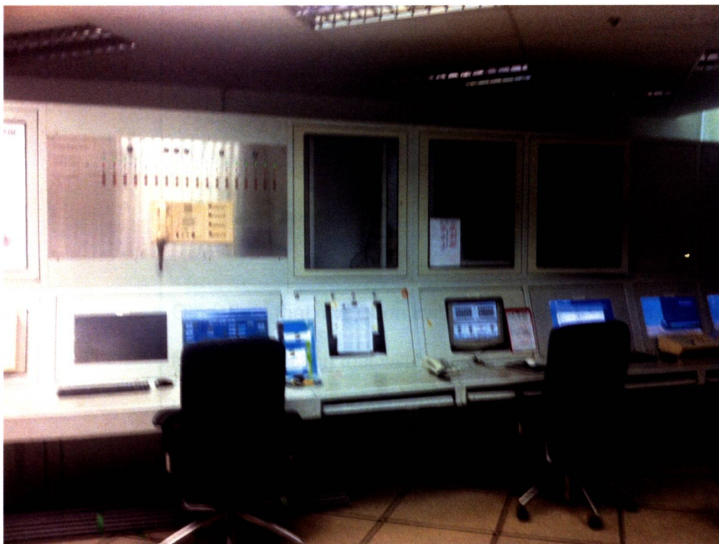
Figure 5: Control room (Ministry of Federal Territory). Level G.
