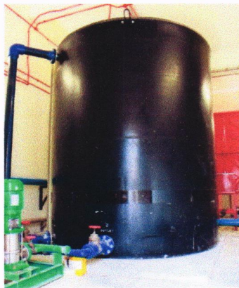
Figure 5.4.6: Inside water pump room
