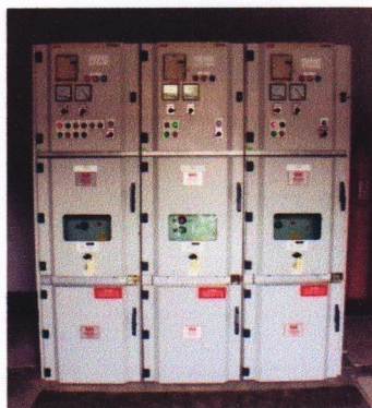
Figure 5.4.2: Switchgear at Substation New Library
