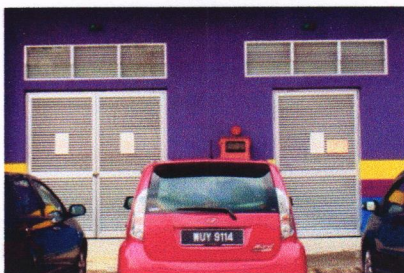
Figure 5.4.1: Substation of New Library
