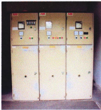
Figure 5.2.2: Switchgear at Substation No 1
