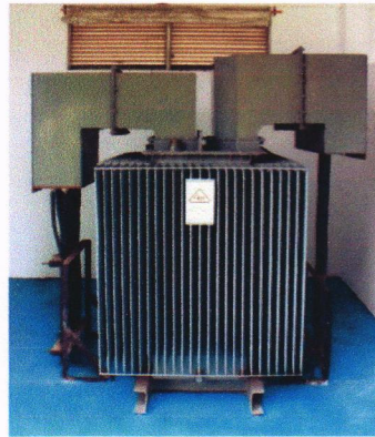
Figure 5.3.3: 1500kVA Transformer Substation No 2
