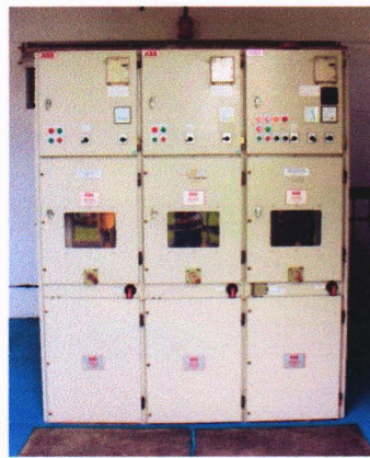
Figure 5.3.2: Switchgear at Substation No 2
