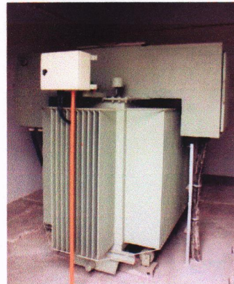
Figure 5.4.3: 1250kVA Transformer Substation New Library
