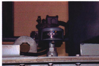
Figure 5.2.5: The transformer increase in temperature
