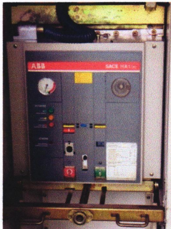
Figure 5.2.7: 11kV 25kA Gas Insulated Circuit Breaker Substation No 1
