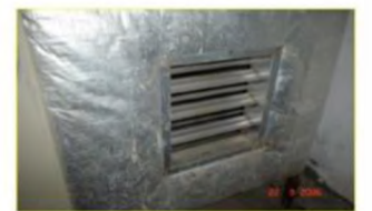
Air Handling Unit (AHU)
