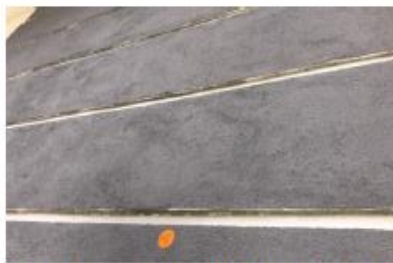
P62- Uneven paint surface on the wall
