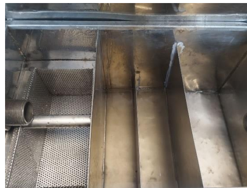
Plates 3. 1 Restaurant Wastewater in Grease Trap
