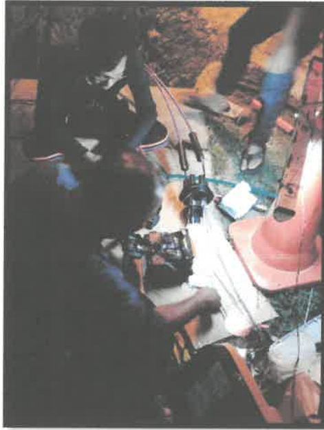
Figure 3.1.5(d) : Observation of connecting broken fiber cable
