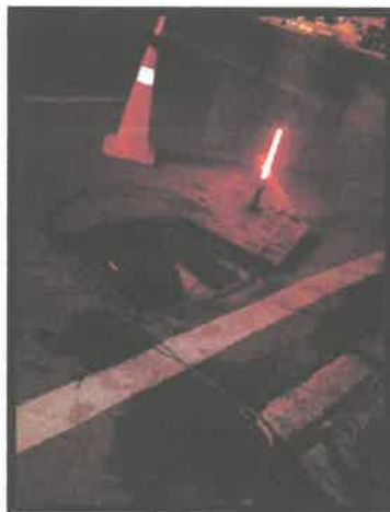
Figure 3.1.5(c) : Safety cones are place to aware the road user from the maintenance work on the main hole
