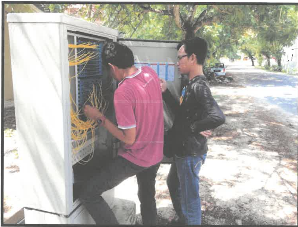
Figure 3.1.6 : Checking the connection available on the network cabinet at Kubang Kerian
