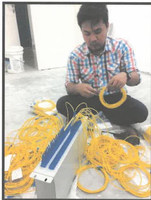
Figure 3.1.5(e) : Installation and design the fiber cable arrangement to the network server
