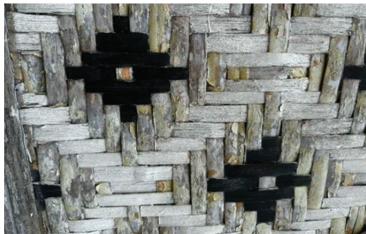
Figure 3. Current condition of the kelarai walls of Ihsaniah Iskandariah Mosque, Padang Rengas
