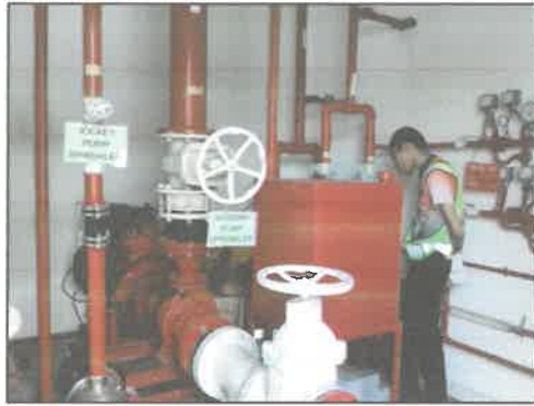
Figure 3.44: Water pump engine checking.
