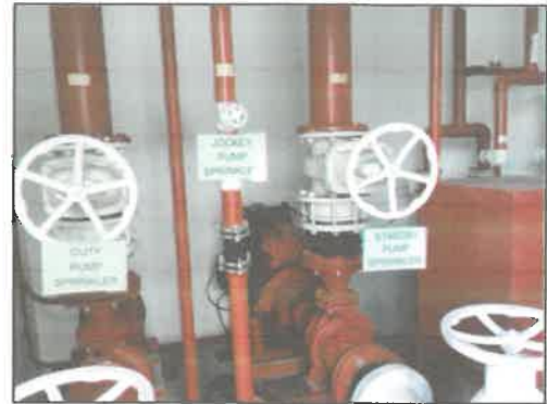
Figure 3.45: Water sprinkler pipe.
