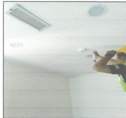
Figure 3.47: Smoke detector checking.
