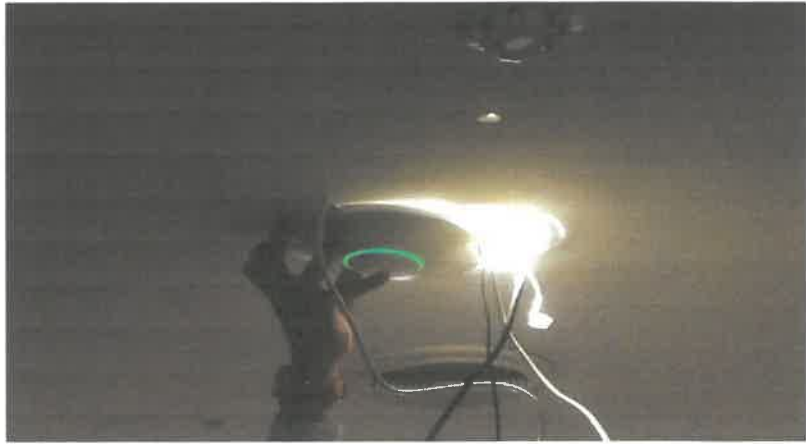
Figure 11: Ubiquity Devices at level 10
