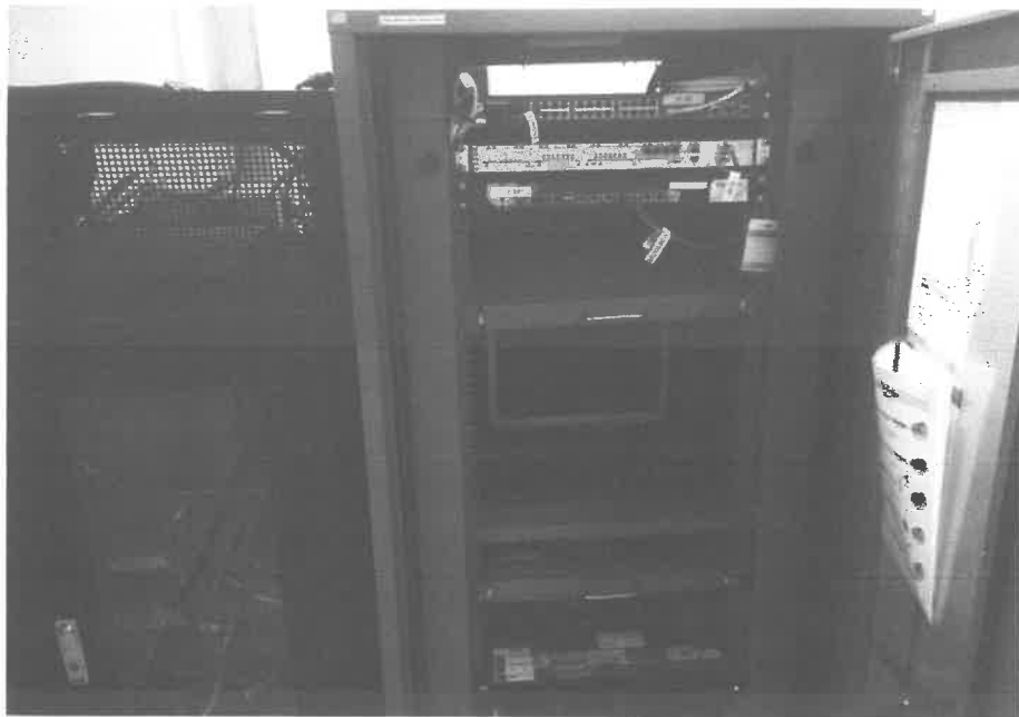
Figure 47 : Server Rack at PPD Muar
