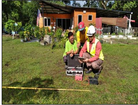
Figure 2. Sub-surface soil layers can be identified early on using a geological scan or geomap
