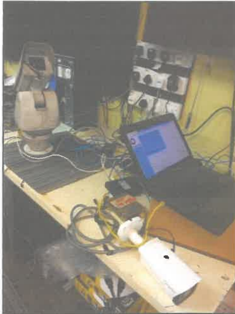
Figure 9: CCTV configuration before testing
