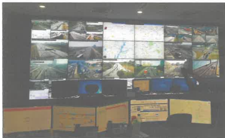
Figure 6: BESRAYA control room
