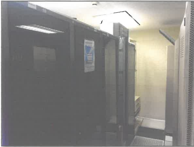
Figure 7: BESRAYA server room
