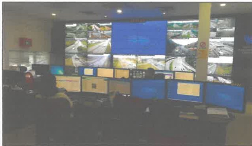
Figure 25: Lembaga Lebuhraya Malaysia (LLM) control room
