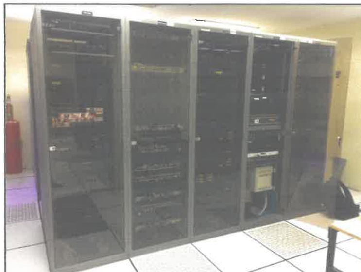
Figure 26: Server room in Lembaga Lebuhraya Malaysia (LLM)
