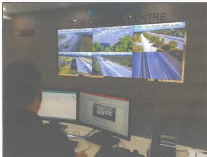
Figure 23: View in SKVE Control Room
