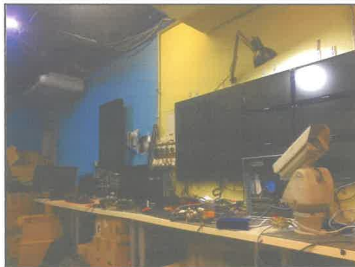
Figure 8: CCTV testing room at Phileo Damansara
