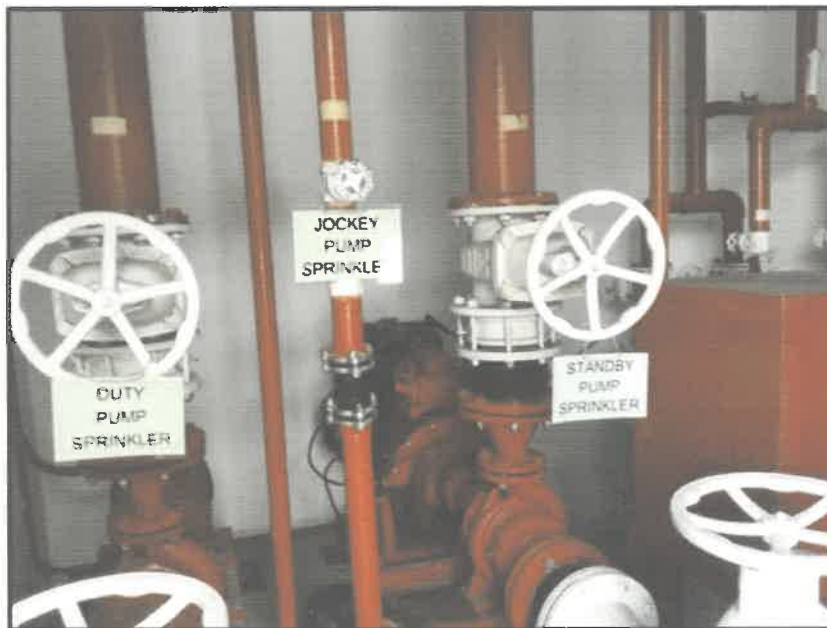
Figure 3.1.8 (a): Water sprinkler pump
