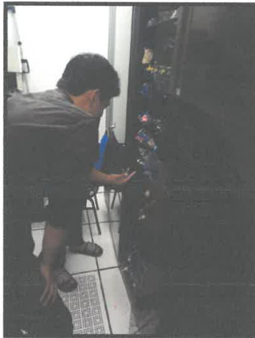
Picture 23 : Server room
