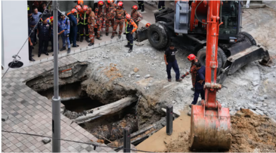
Figure 2: Sinkhole case on Jalan Masjid India, Kuala Lumpur
