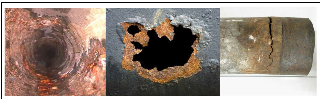
Figure 1.1: Corrosion defects of subsea pipelines (Meruonline, 2023)
