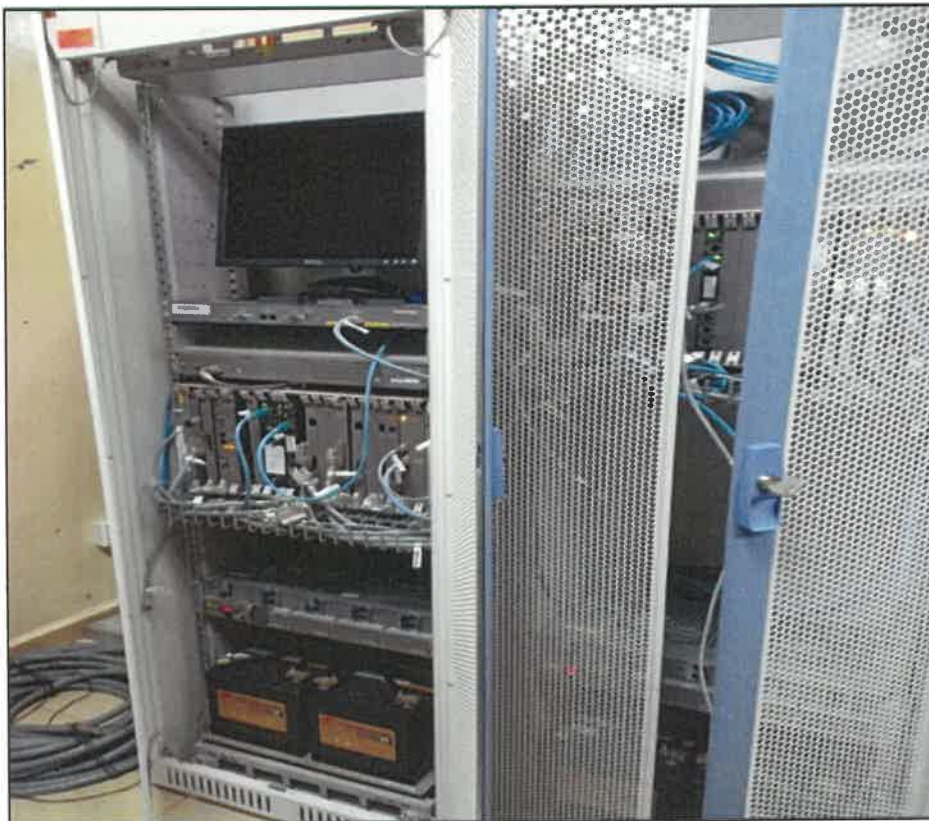
Appendix 68: The wired rack that was connect with 3000 extension wired
