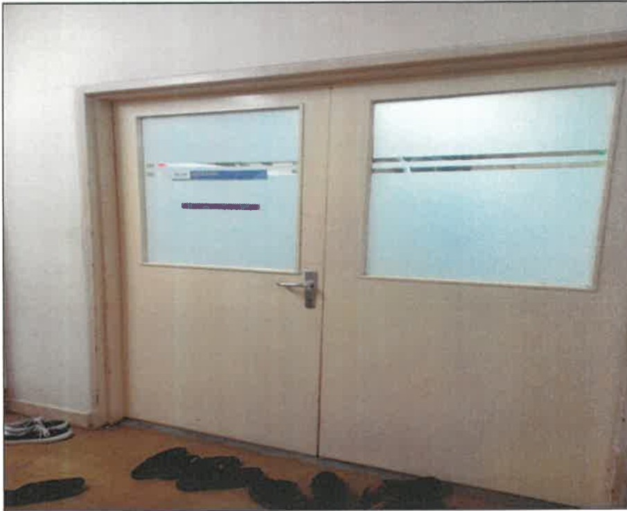
Appendix 67: An entrance door of PABX room
