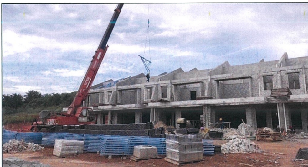
Figure 3.6: Mobile crane lifting up the bundle of truss to the roof beam
