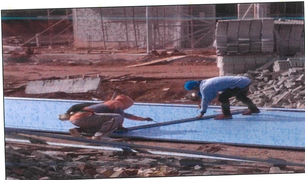
Figure 3.4: Workers are measuring and marking the length required on the steel truss
