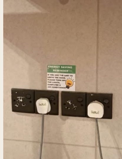
Put an Energy Saving Reminder on each switch at Level 9.
