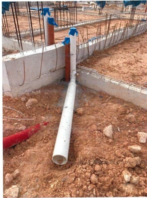
Figure 23 Rainwater Down Pipe
