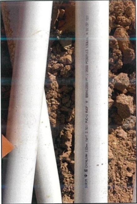
Figure 12 Rainwater Down Pipe
