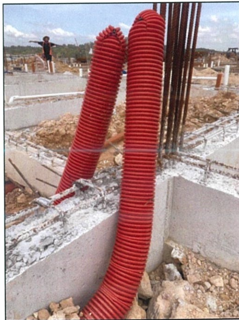
Figure 14 Corrugated Electrical Pipe
