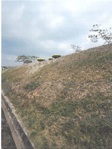
Figure 3.19 : Slope damage at SSTMI
