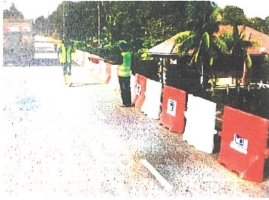
Figure 3.2 : Plastic barriers placed along the road (Source: Courtesy of JKRKT)
