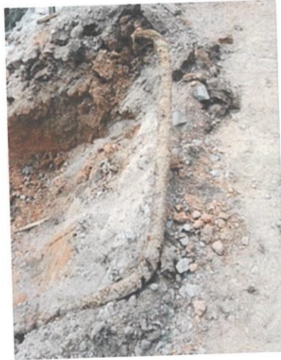
Figure 3.4 : Electric cable found beneath the ground
