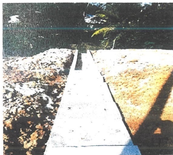
Figure 3.15 : Concrete slab as the cover for toe drain (Source: Courtesy of JKRRKT)
