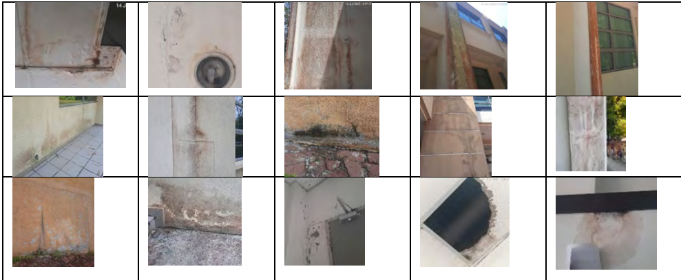
Figure 2: Visual Mould found on Quantity Surveying Building
