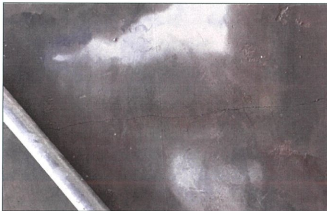
Figure 3.12: Example of crack.
