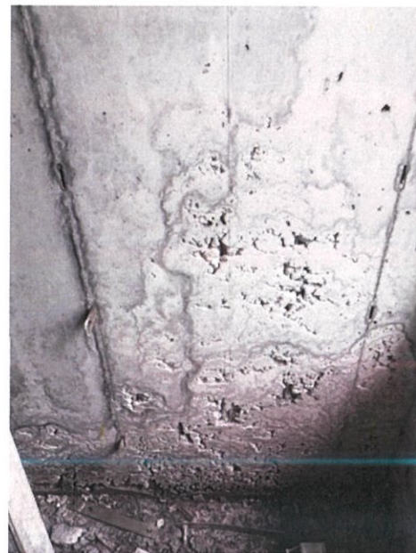
Figure 3.10: Example of Minor segregation
