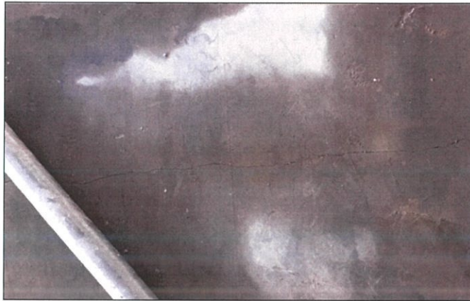
Figure 3.37: crack line at carpark RC slab
