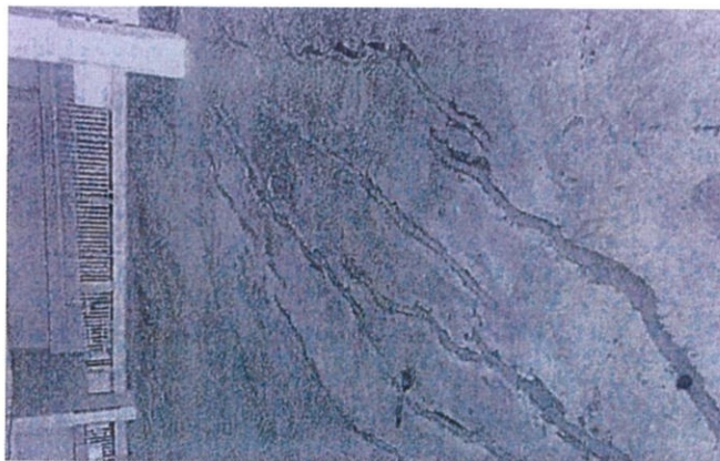
Figure 3.40: grout was settled
