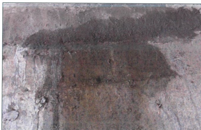
Figure 3.43: crack leakage at rc wall
