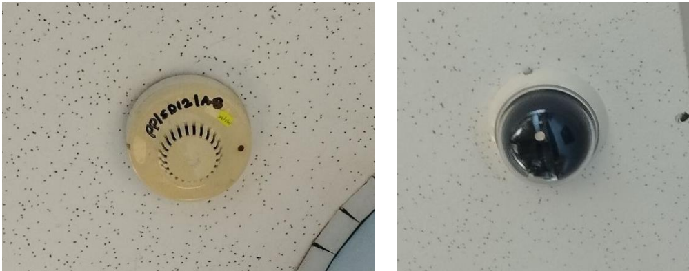
Figure 22: Smoke detector & CCTV
