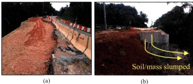
Fig 2 : Site visit Km 16 Panching – Sg. Lembing: (a) View from on road after landslide, 2015 (b) soil or mass under the road rotate and slumped down.
