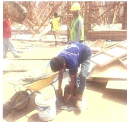
Figure 26: The worker does not wear a proper Personal Protective Equipment (PPE)
