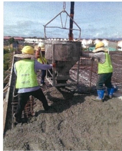
Figure 23: The workers handling the concrete bucket lifted up by the crane for the first floor beam
