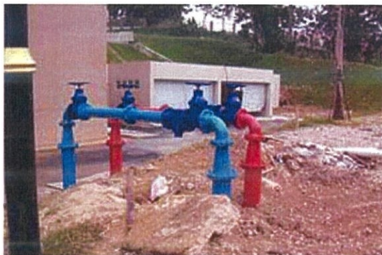
Figure 3.12: Water Meter (blue) & Hydrant Meter (red)
