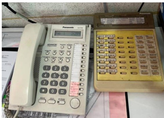
Figure 10: Office's Communication System
